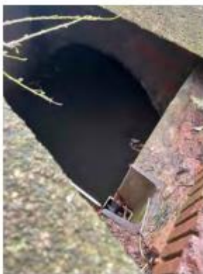
SW2 UPSTREAM HOLDING HIGH WATER LEVEL
