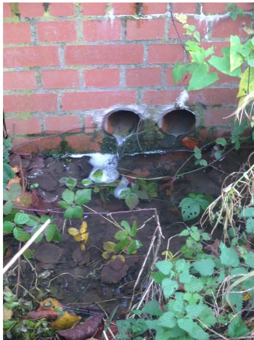
Figure 19 Discharge of Runoff Water into Adjacent Watercourse
