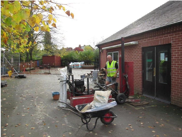
Photo depicting the 'Competitor' Windowless Sampling Rig drilling WS5 within the current car-parking compound, around the perimeter of the school building.
